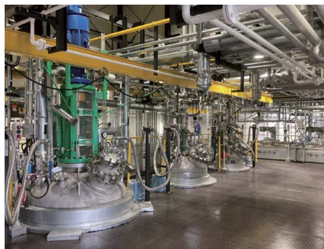
Waterborne resins production facility (Japan)
